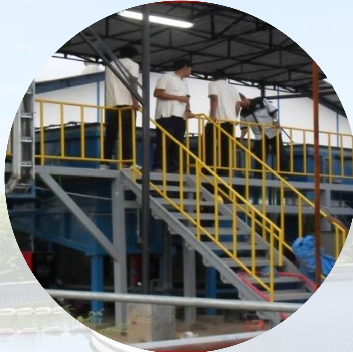
Consultant and Contractor Water and Waste Water Treatment Plant
